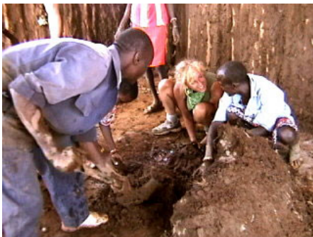
Mixing the mud, water and cement for the walls of the school.
